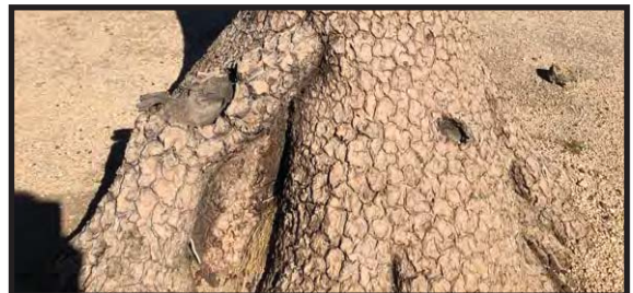
Image 1: Holes at large branch joint
