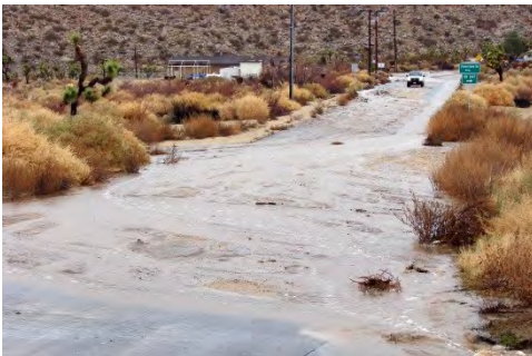
Floodwaters inundating a low-lying roadway.
