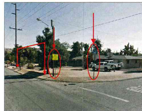
NEC of Sage Avenue at Pueblo Trail. Proposed sidewalk will be constructed alongside the existing berm. NEC return terminates at BCR on Pueblo. Some signage relocation may be required.
