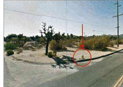
SEC of Sage Avenue at Pueblo Trail. Sidewalk and returns to be constructed along Sage, and corners terminating at ECR on Pueblo. Design requires protection of existing hydrants.
