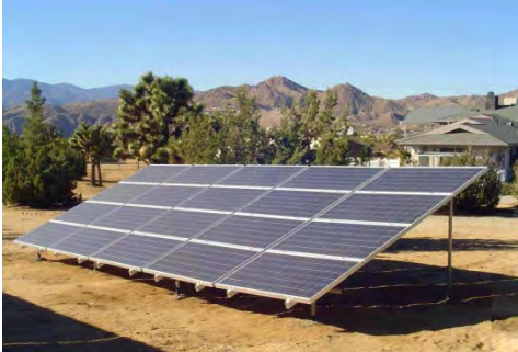
An example of ground-mounted solar panels in Yucca Valley.
